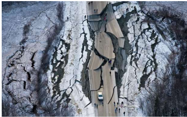
Vine road embankment, 2018 Mw 7.0 Anchorage, Alaska
