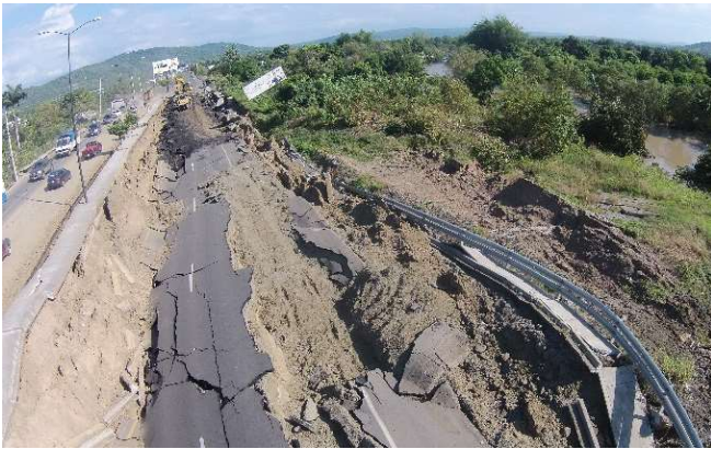
Mejia embankment, 2016 Mw 7.8 Pedernales, Ecuador
